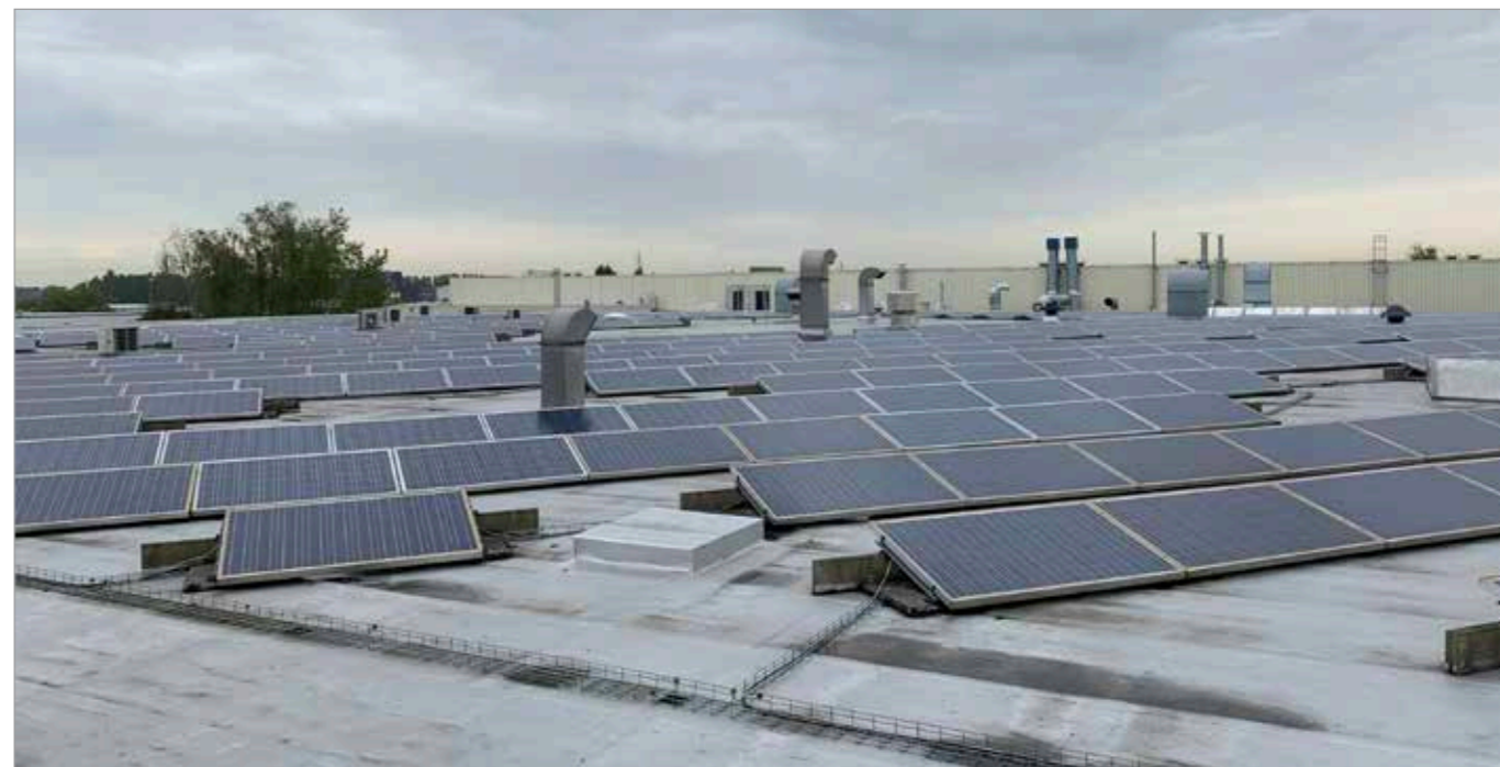
Solar voltaic panels at our manufacturing plant in Belgium
